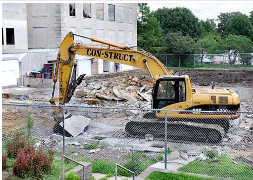
Crews spent much of the summer disassembling the old horticulture greenhouses so the components could be recycled or reused. Photo by Bob Elbert.
