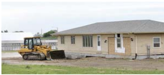
Atop a new basement, the house awaits renovations. Photo by Bob Elbert.
